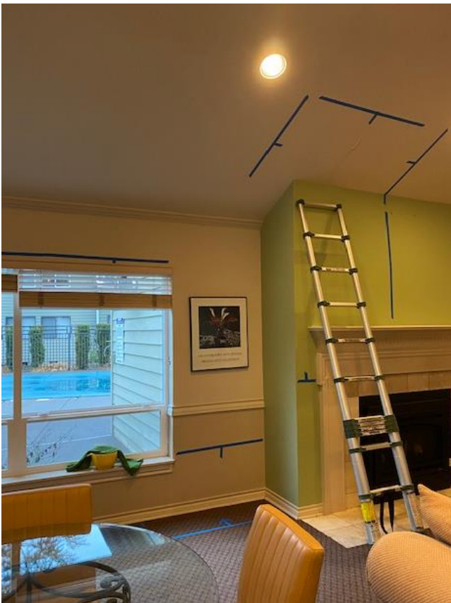
A slow roof leak has caused damage to the Fireside Room. It is being repaired. Thank you, Leanna, for letting us know about the drip drip, DRIP!
