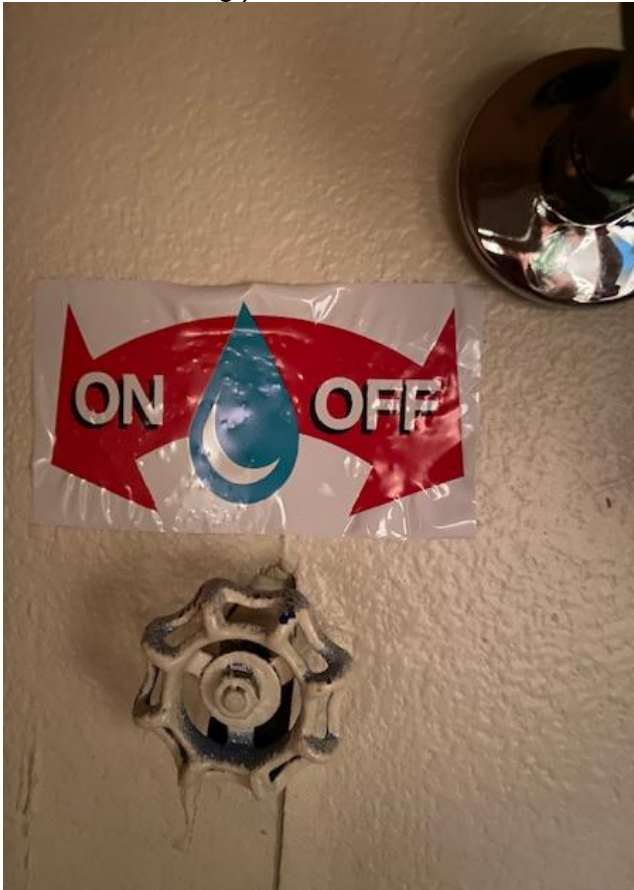
This is the turn off valve for your individual unit. It is under the sink in the guest bathroom.
