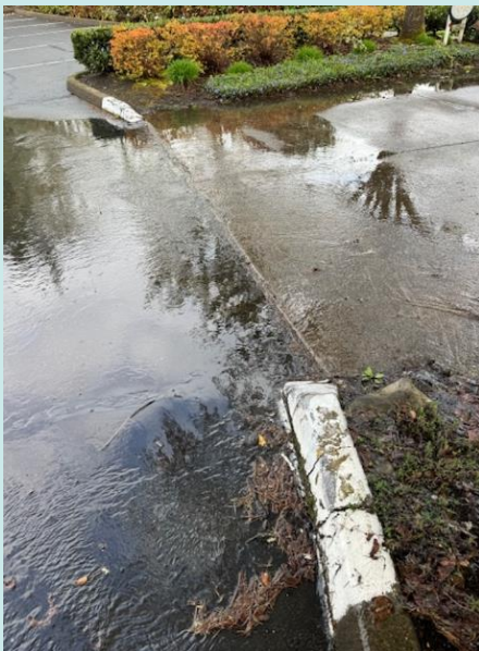
Irrigation leak at OPV!
